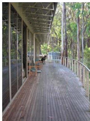
Exposed timber should be treated with fire retardant.
