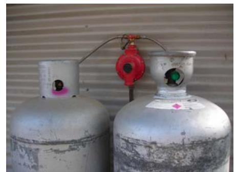
These LPG tanks are stored away from the house. Vents are facing away from the wall.
