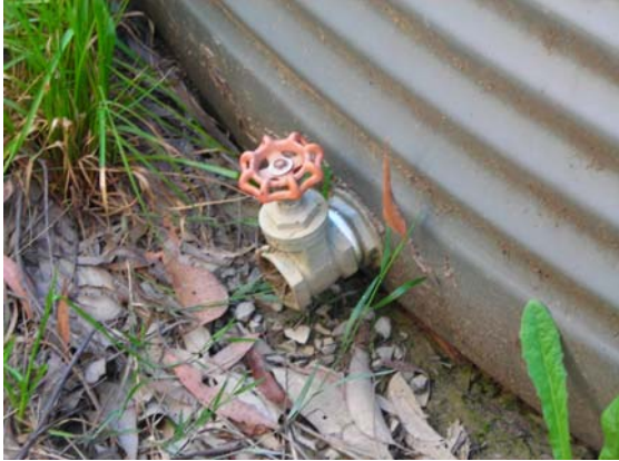
This water tank fitting allows fire brigade access.
