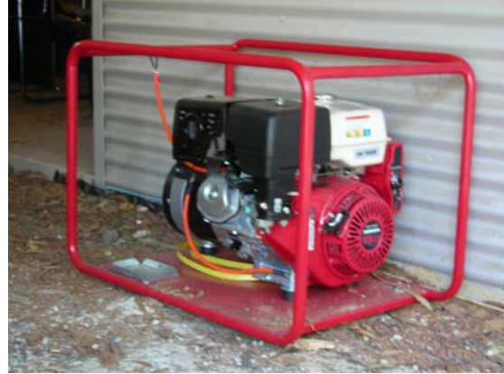
A diesel fuelled generator provides power for the water pump to operate in the case of fire.
