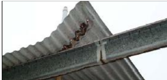
Corroded screws and cladding
