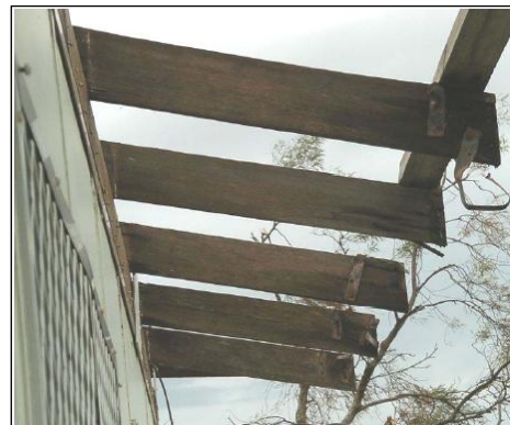
Corroded batten straps
