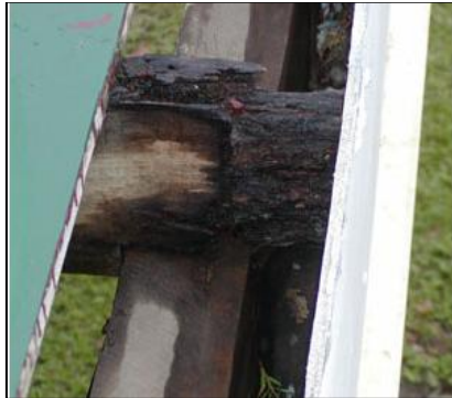
Deteriorated timber (Floor joist at external wall connection)
